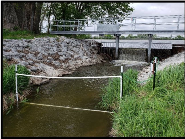
PIT Monitoring Station Setup at the Clear Lake Outlet.
